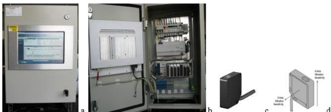
Fig. 3 –Equipment of the HolderPPS electrical box
