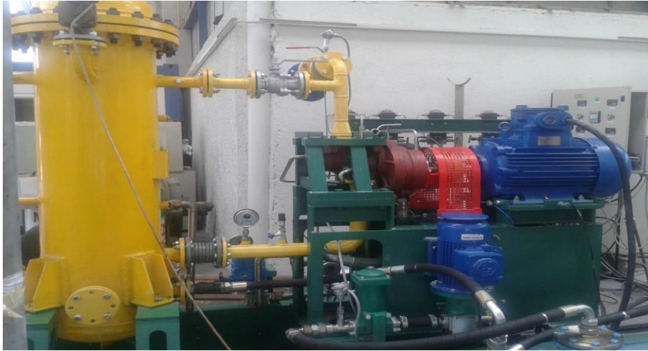
Fig. 3 The testing stand from COMOTI includes the 37kW expander– asynchronous electric generator skid
