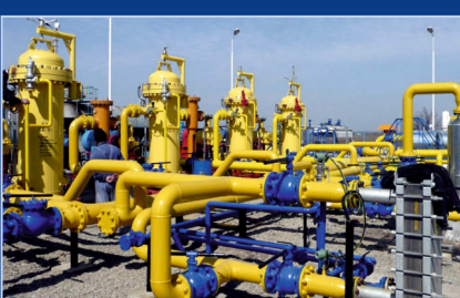
Screw compressor skids station.
