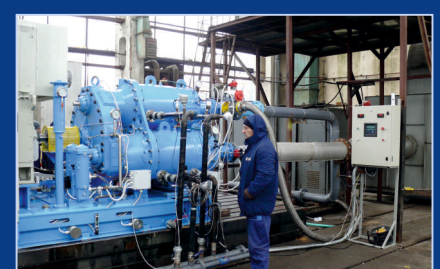
Centrifugal compressor skid.
